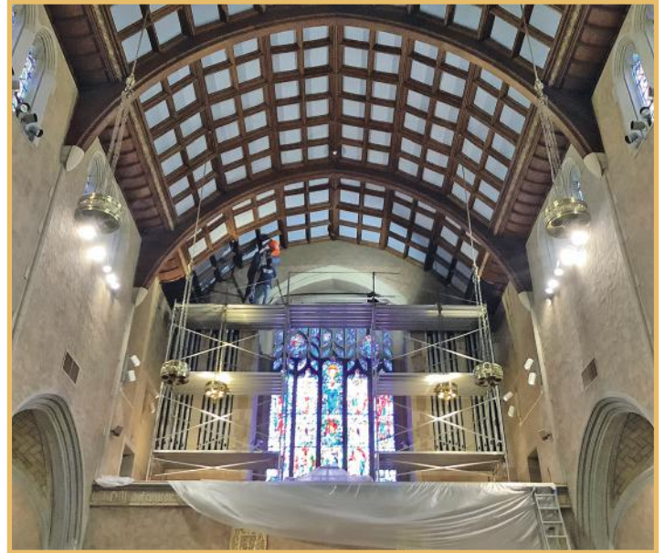
The week of August 31, work began on cleaning the walls in the choir loft.
