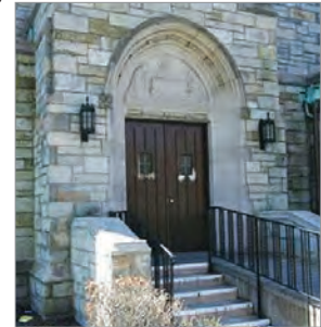
Queens Blvd. double doors require renovation
