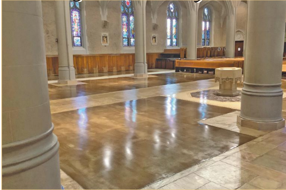
Middle section of the refinished church floor, before the pews are put back in place. Report on page 4.
