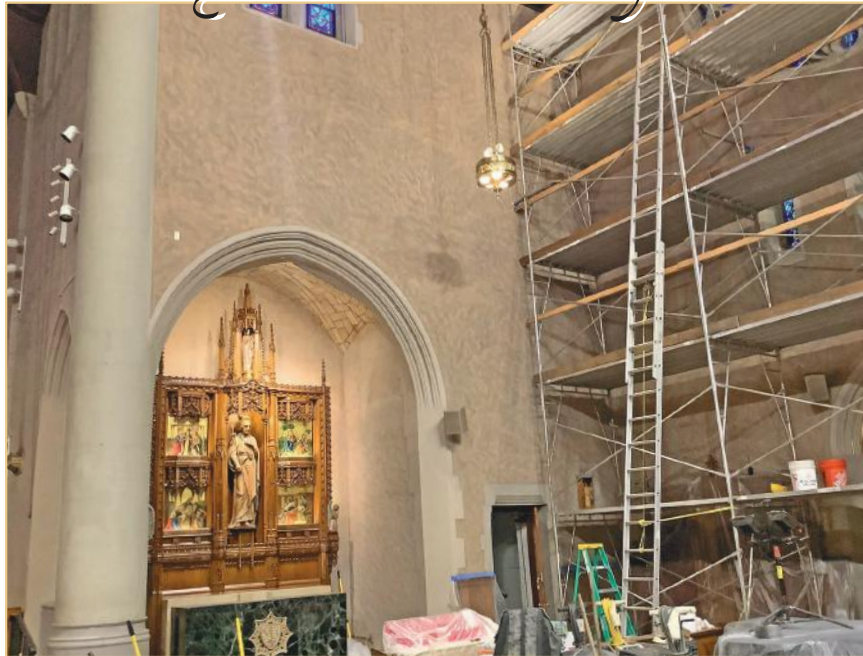
The completely restored wall at the St. Joseph's Altar. See Major Repairs Report #5 on page 4.
