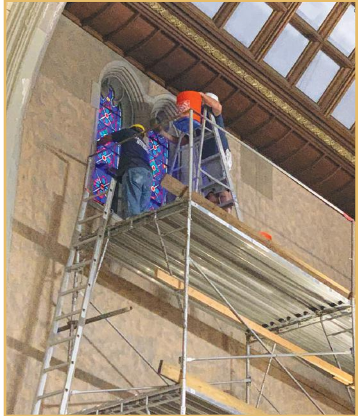
Before and After—Wall above the St. Joseph Altar. Notice the untouched areas near the ceiling molding (dark square on the right and area left of the stained glass window).
