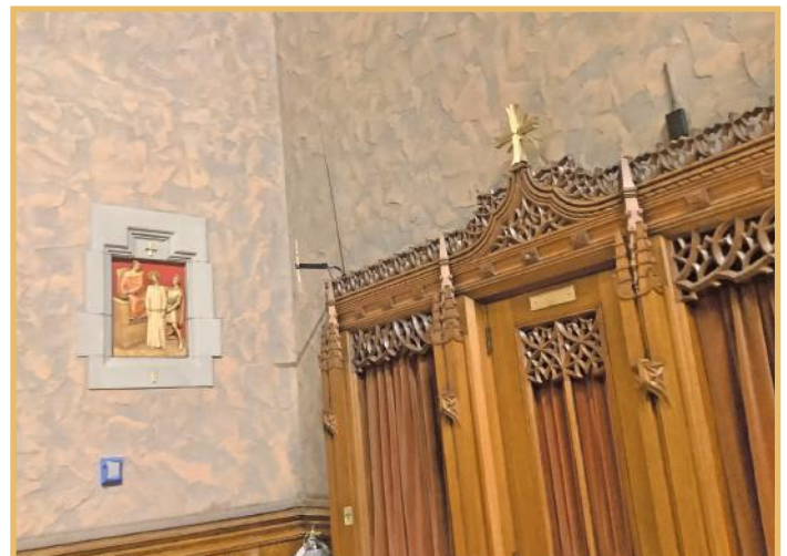
Pictured— The church's interior walls are cleaned and brightened, including the Stations of the Cross artwork on the walls.
