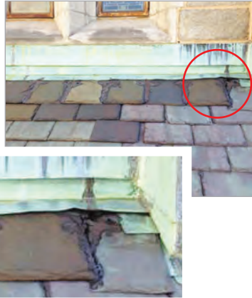
Shown here is a section of the lower Church roof, school side, that is in need of repair to prevent water penetration and damage to the interior
